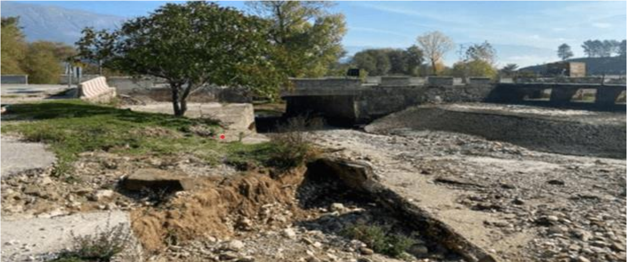
Figure 2: Overview of the bridge and the damage to the bed.
